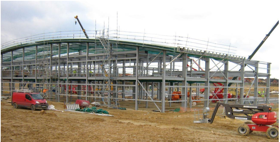
Data Centre – Norwich Union
