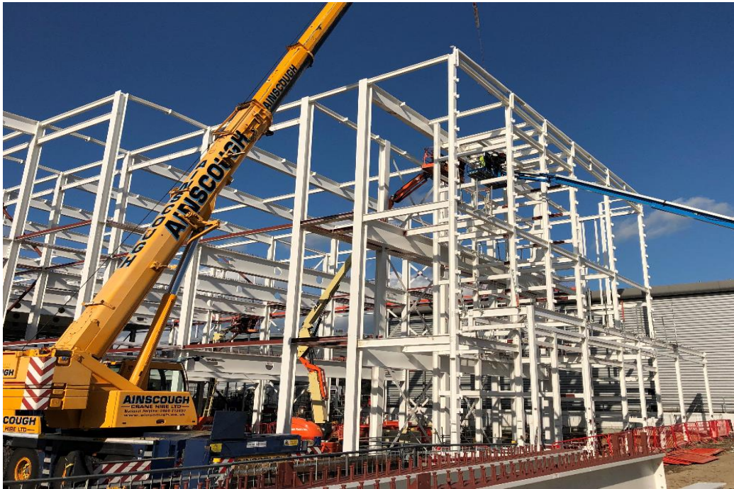
LD11 Equinix Data Centre, Slough
