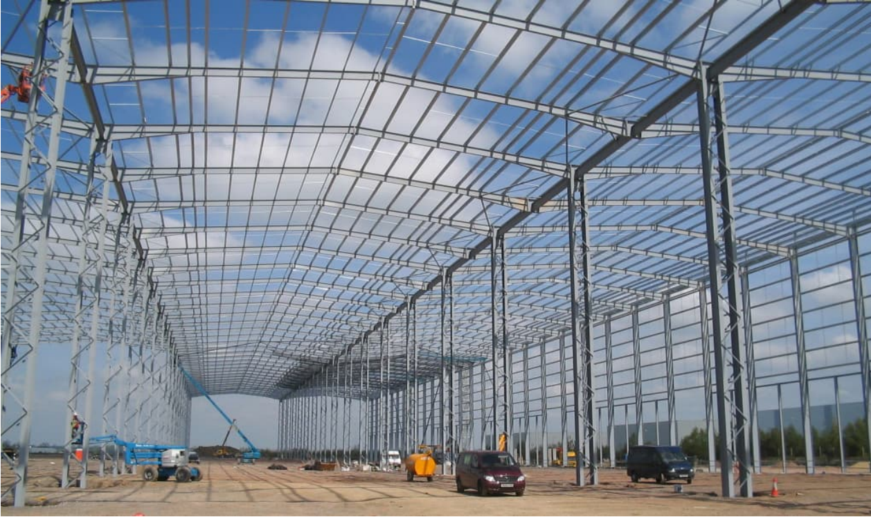
Distribution Facility, DIRFT Central - Northampton
