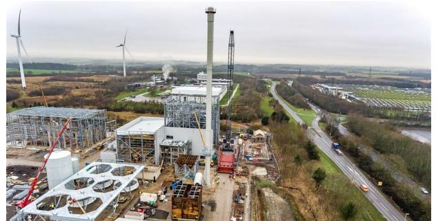
(BWSC Biomass Plant - Cramlington)
